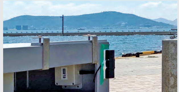
Case study: open/close monitoring of a tsunami water gate
